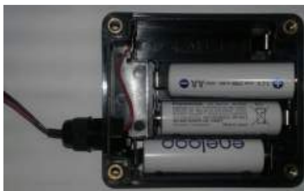
Fig. 21 – Replacing battery in battery box
